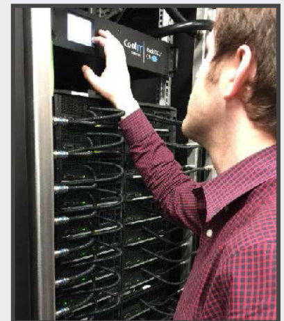
Data Center using Rack DCLC™ CHx40
