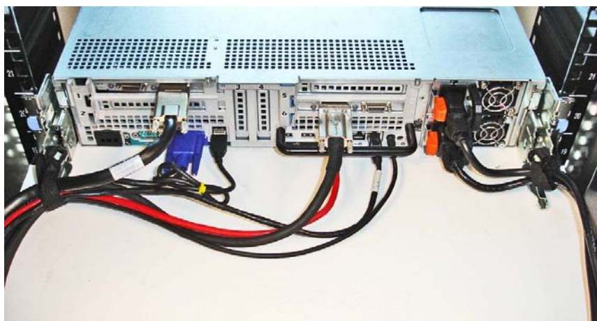
Figure 6: Cable Routing Without a CMA
