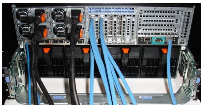
Figure 1. System with cables installed
