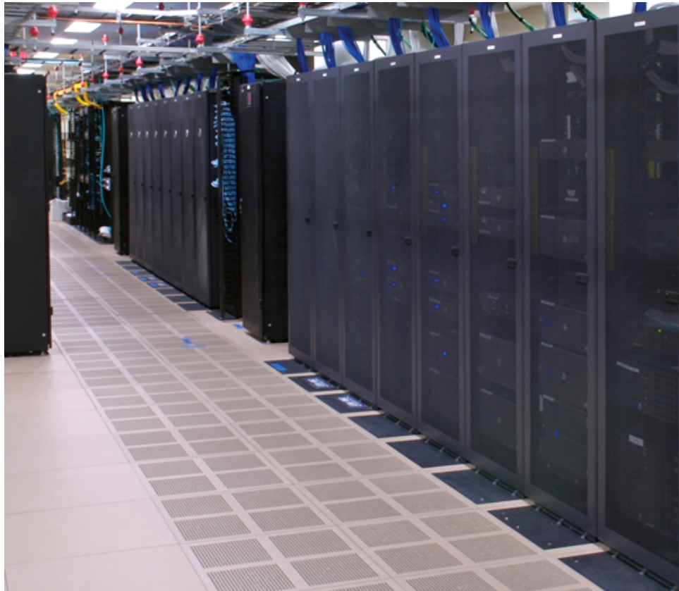
Figure 1. Typical Data Center
