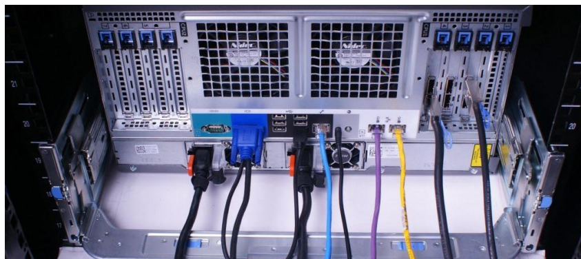
Figure 1. System with cables installed
